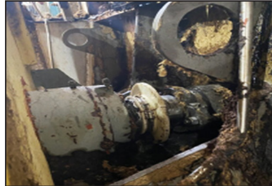
Equipment before AMPS unit installation. It was very difficult to access bolts to make any adjustment, and unsafe to do while running.
